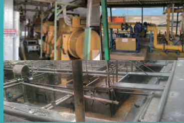
Palm Factory Waste Liquid (POME) Power generation business (Indonesia Sumatra)
